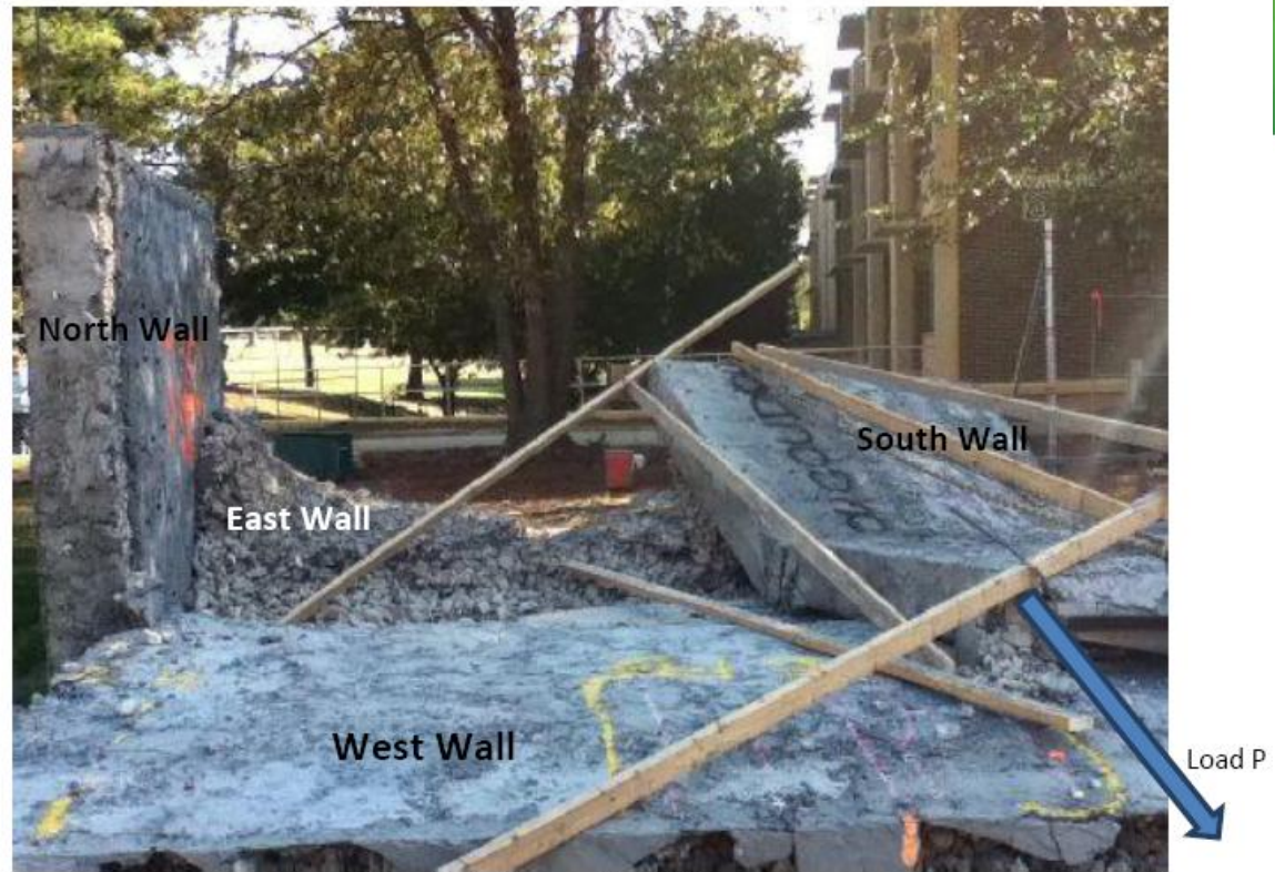
(a) Rubble-House after failure
