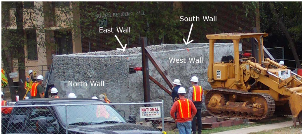
Figure 1 Rubble house built next to a student residence building.
