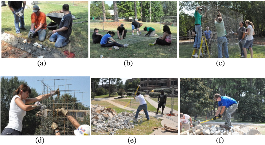
Figure 5 (a ) Student volunteers working on foundation installation, (b, c, d ) preparing wire baskets, (e, f) busting concrete.
